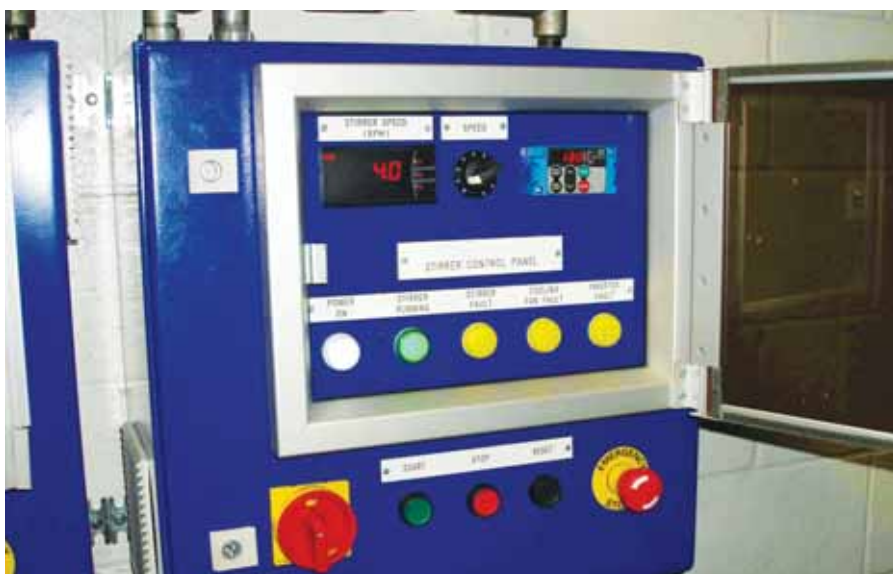
▲ Stirrer control panel.
