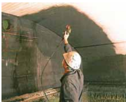
▶ Fig 2. Spraying a high emissivity coating on the crown of a furnace.
